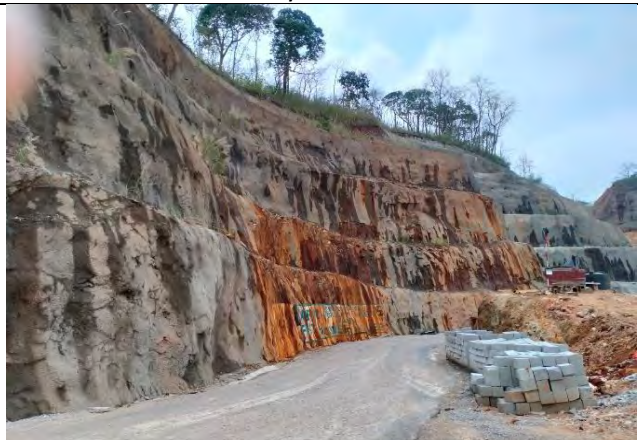
Possible Pyrite Prone area at Power House near the Side Way
