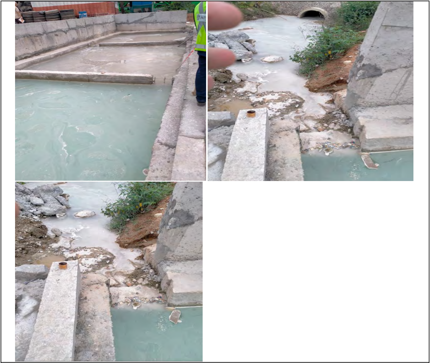
Sedimentation tank constructed to collect the discharge water from the Batching and additive units of CP-2 contractor.
