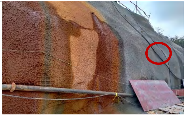
Sample 3 (PH2) from the point just beneath E-130 at Power House near the side way
