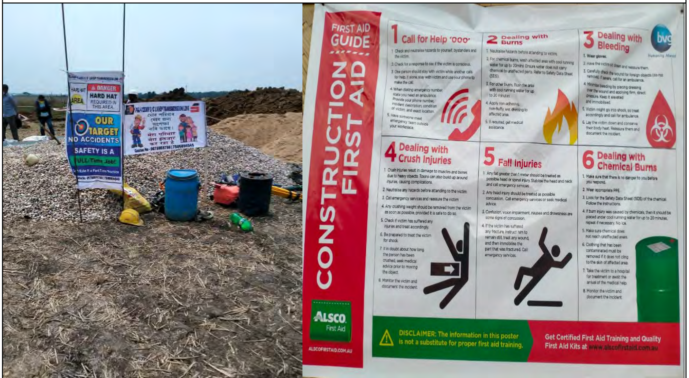
Display of Emergency contact and Safety Signages
